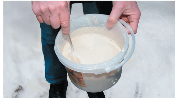
2. Immediately after sifting, start mixing plaster with water in the mixing pail using a spoon. Stir until the mixture starts thickening (45 - 60 sec).
